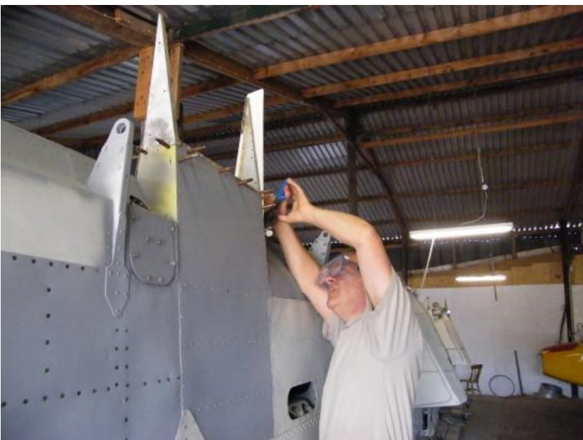
Mark Porter installing skin clips to secure smaller skin sections to the trailing edge of the port outer wing lower surface.
