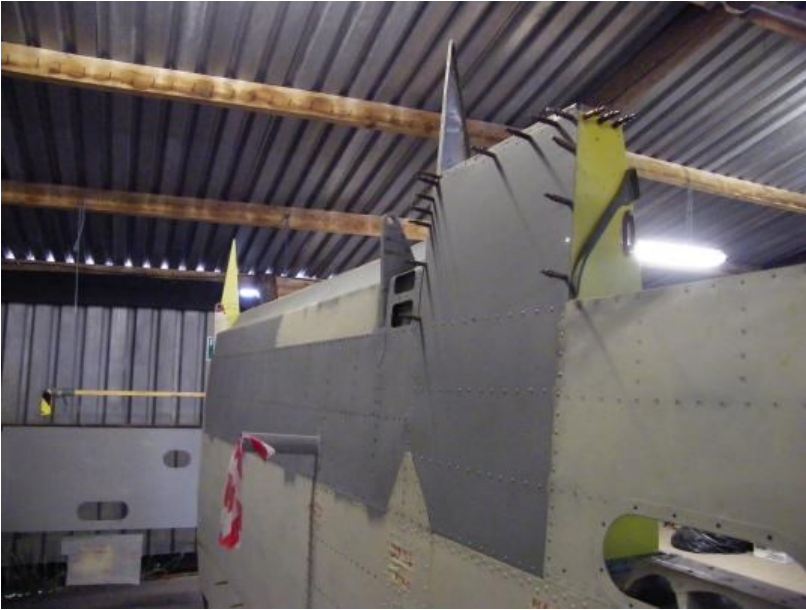
View of the fixed section skin panel (between the flap and the aileron) is in the process of being re-installed.
