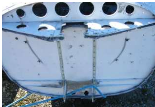
Frame 19 with nose wheel mounting structure missing.
