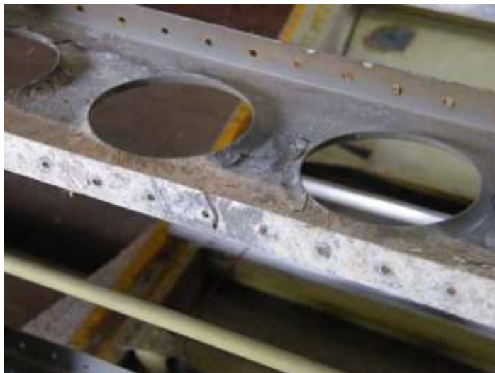
Corrosion and damage to frames and longerons in underfloor structure.
