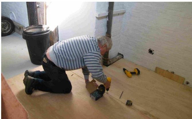
BNAPS Trustee and Engineering and Operations team leader Bob Wilson puts the finishing touches to the new floor on 1 March 2012.
