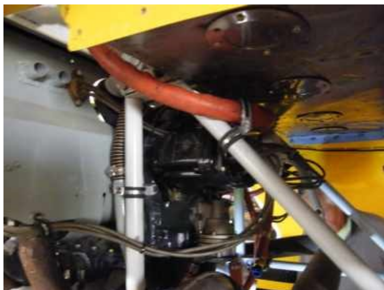
View of the port engine rear section where fuel hoses and other items are located showing the confined work space.
