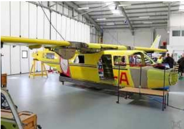
In Hangar 6 Islander G-BKJM, c/n 2162, was undergoing a major rebuild and had reached the stage where the wing and fuselage would soon be joined up (BNAPS).
