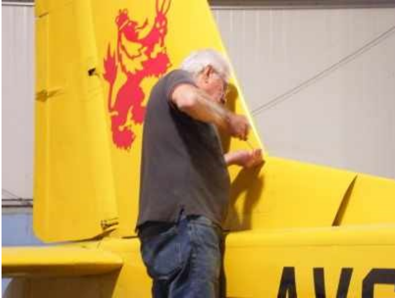
Bob Wilson installed a detail fairing section at the junction of the fin and dorsal fin.
