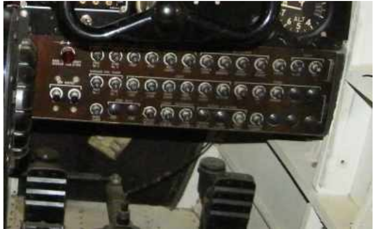
Electrical Circuit Breaker Panel
