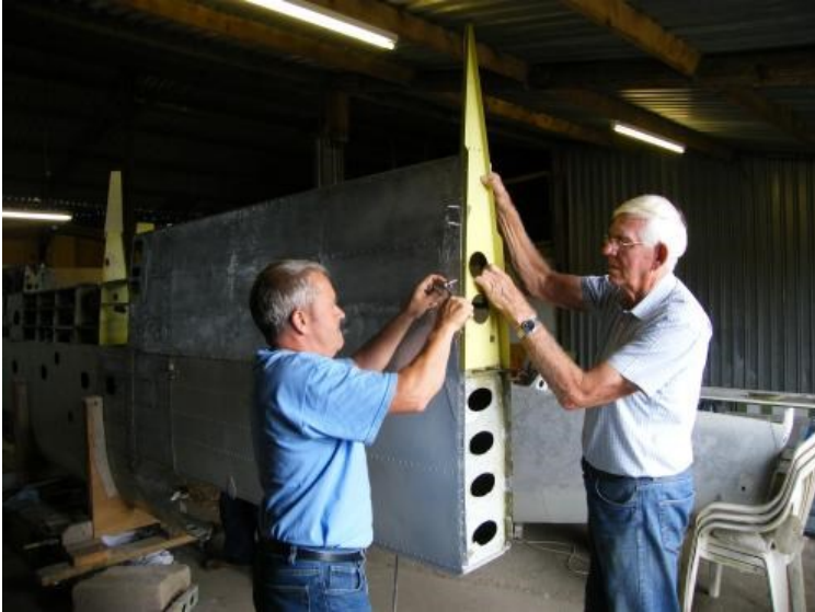
Bob Ward (right) and Mark Porter undertake a trial installation of a new rear bay end, the wing tip will be attached at a later stage
