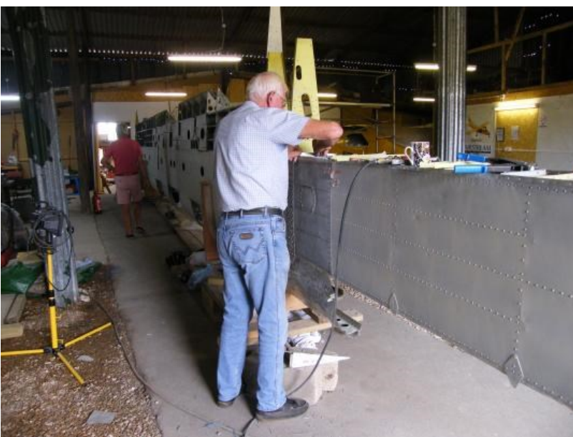
Bob Ward continued with the work associated with attachments for the outboard rear bay section of the wing and installation of a replacement rear bay rib.
