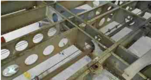
Left: Floor and fuselage under side skin removed for full SB190 inspection.
